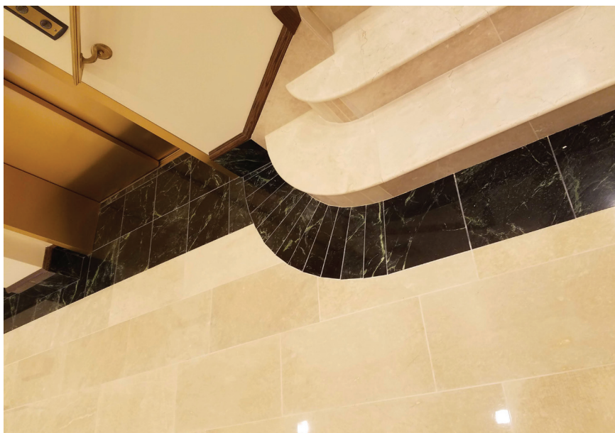
WTG installed 12"x12" and 12"x24" Back Bay Limestone Allura Crema Polished floor tile, with a 12"x12" Daltile Marble Empress Green Polished tile border and base. Credit: WTG Terrazzo.
