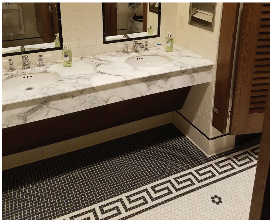
The walls were installed with US Ceramics U974 Biscuit field tile, with two ¾"x6" liner bar accents, using US Ceramics U759 Black and a 2-1/2"x6" Victorian Rail in US Ceramics U759 Black. Credit: WTG Terrazzo
